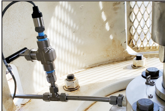
P/T sensor in a two-stage vertical turbine booster pump.
